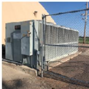
Sternberg Meseum Chiller Replacement R&R Funding
