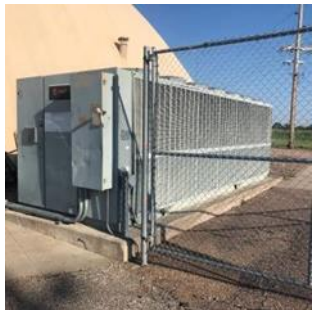
Sternberg Museum Rehabilitation & Repair Funding Chiller Replacement
