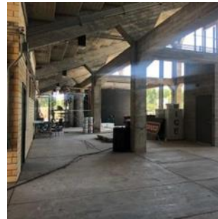
Lewis Field Rehabilitation & Repair Funding New Restrooms for men and women at the West Stadium
