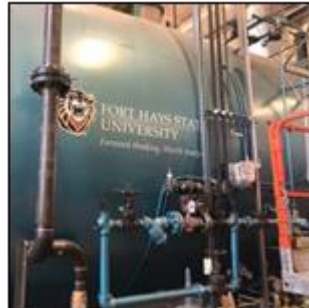
Akers Energy Center Rehabilitation & Repair Funding Boiler Replacement
